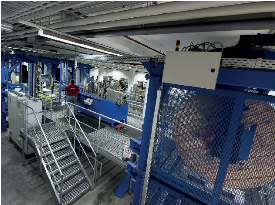
Heavy-load length-cutting facility
